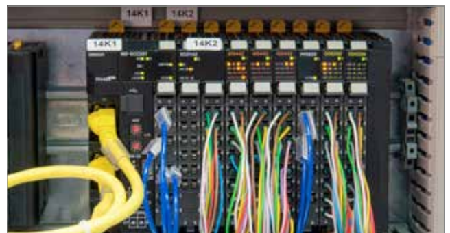
Image 5 Digital I/Os from the new NX series installed in the machine controller.
